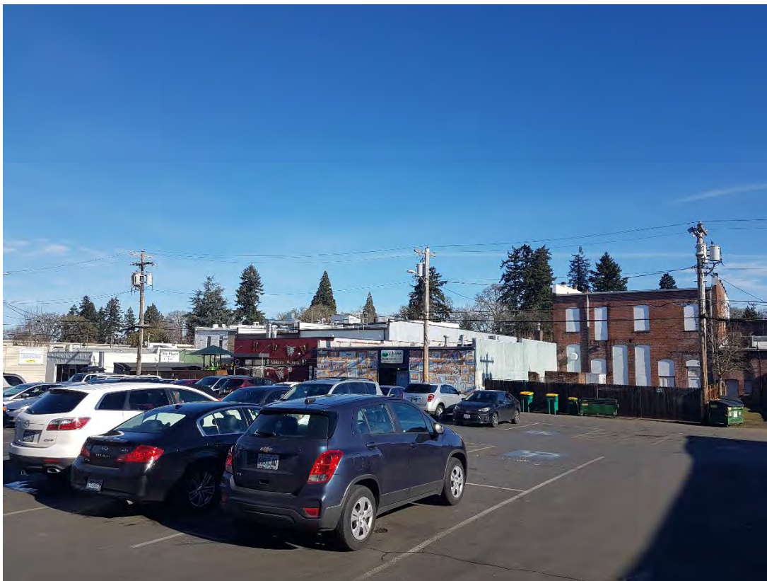
Figure 19: Parking lot #2, with some signs of pavement fatigue and striping fading emerging
