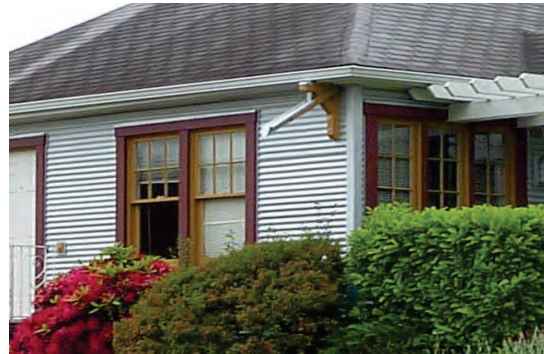
Example of an Inappropriate Siding Revision
