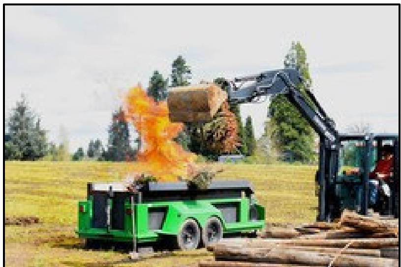
Above: An air curtain incinerator getting loaded with wood waste. Photo courtesy of Clean Water Services
