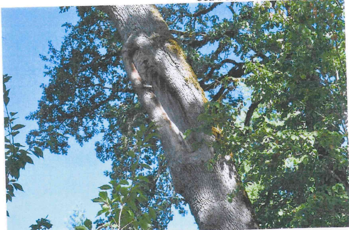
Tree 1 with old scar from prior large stem failure.
