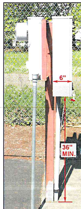
Figure 13: Freestanding CT Meter Base
