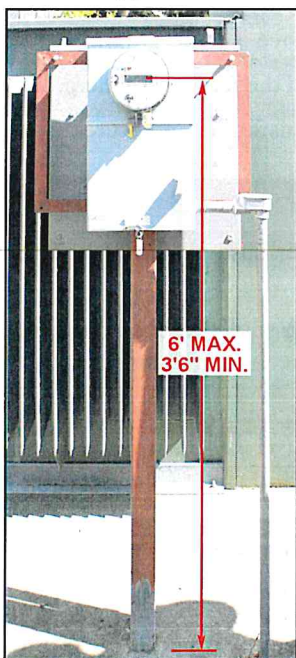
Figure 12: Freestanding CT Meter Base
