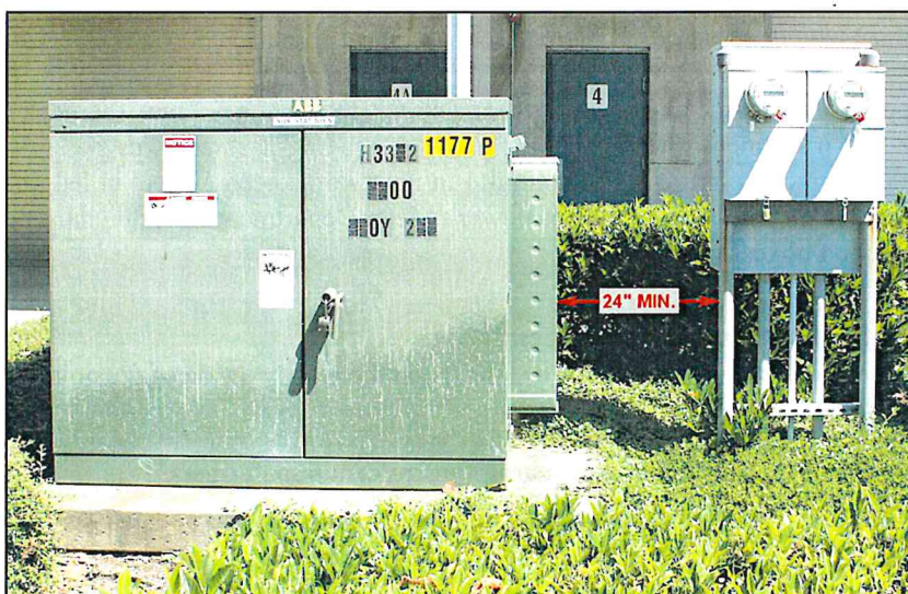
Figure 14: Clearance Between Transformer & Freestanding Meter Base
