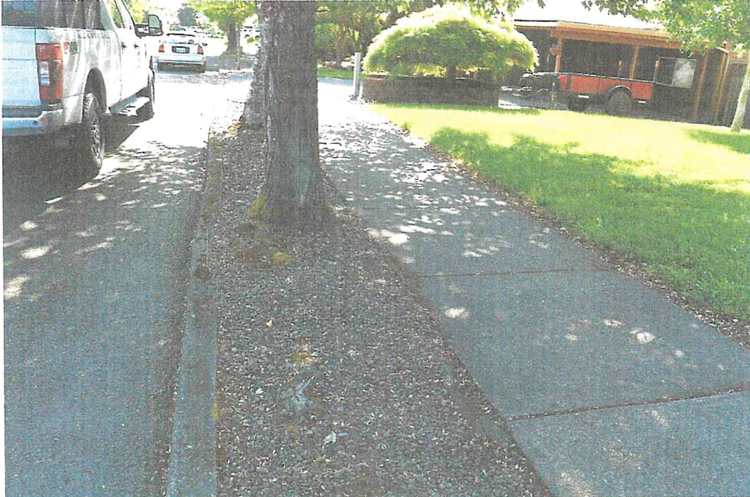
View of how narrow the planter strip is and the west tree and the above ground surface roots. The last concrete pads on bottom are where the roots are lifting the concrete on the lawn side of the pads. Tree scar is also visible on the west side.
